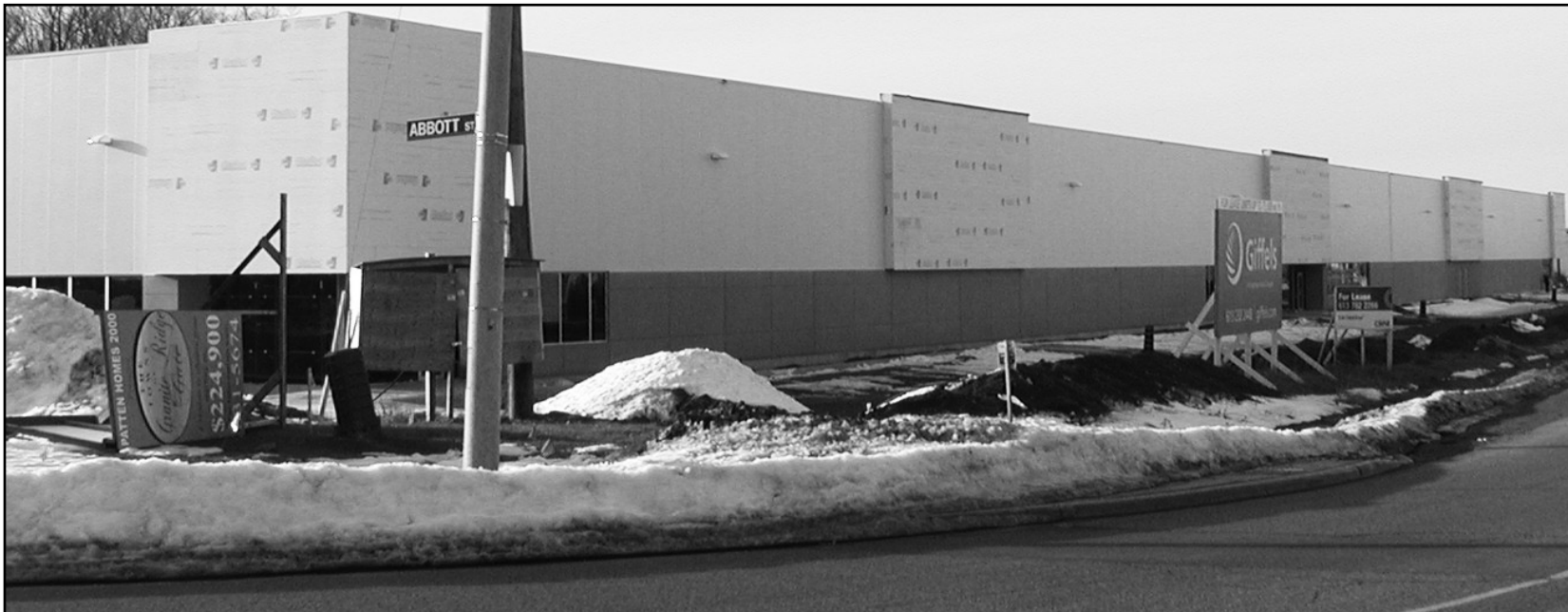
A 7033 square metre multi-tenant industrial building that stretches along the western side
